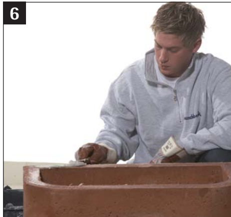
Apply mortar on the upper edge of the base and wood storage
