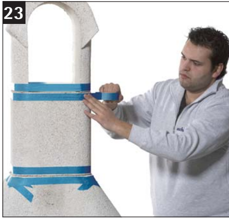
For a neater, finished look, use masking tape above and below the seams.
